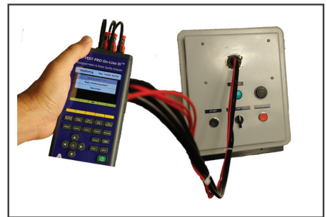
Installed ALL-SAFE inside starter box, connected to ATPOL III™ to start taking readings.
